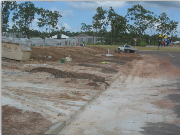
Uncontrolled site access, causing drainage to the verge and sediment discharge to the street, stormwater drainage system and local waterways.
