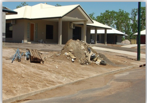
Un-managed soil & material stockpiles
