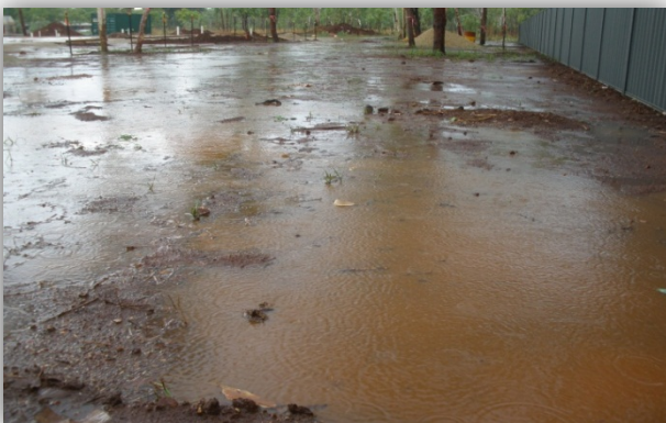
Building site flooded by upslope runoff
